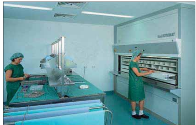
Retrieval of surgical instruments and equipment in the central sterilization room of a clinic
